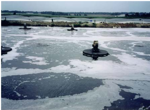
Basin Mixing & Air Distribution (Note: Surface Aerators not in use)
